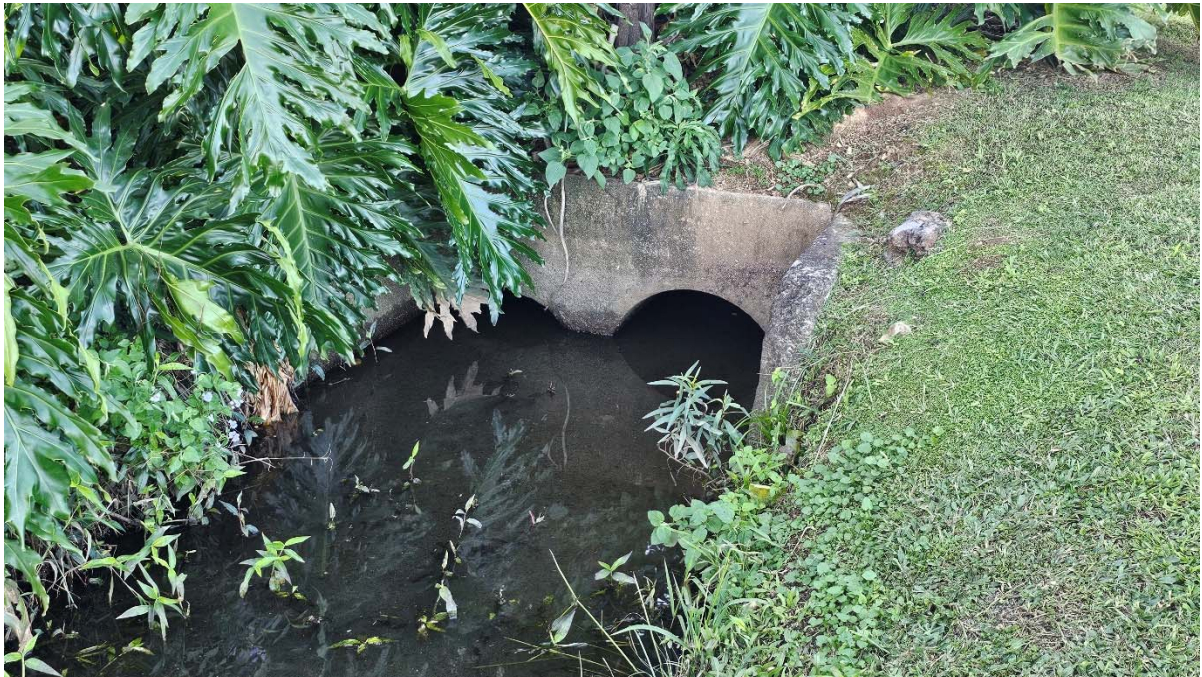
Image 5 - 2x600 Headwall outlet into Left Bank Road swale
